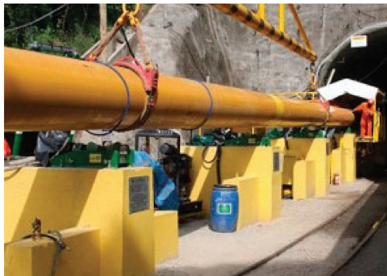
Figure 17: Section of welded pipe string being lifted onto rollers in preparation for being installed in tunnel.
