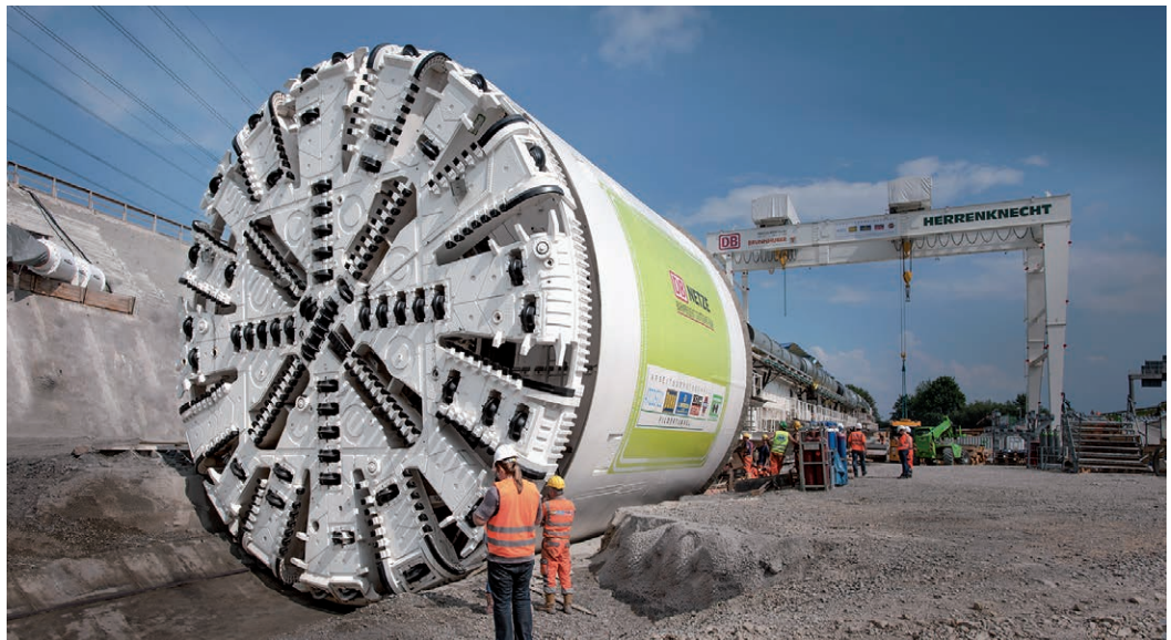
Figure 4: A large TBM—with a 36-foot-diameter cutterhead and shield (foreground) and trailing gear (background) for a total length of almost 400 feet and weight of over 2,200 tons—is readied for the start of construction of the Filder Rail Tunnel in Germany. (Source: Herrenknecht)
